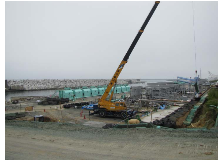
⑫ Maintenance work at port and harbors from Unit 6 seaside yard Sep 15, 2011
