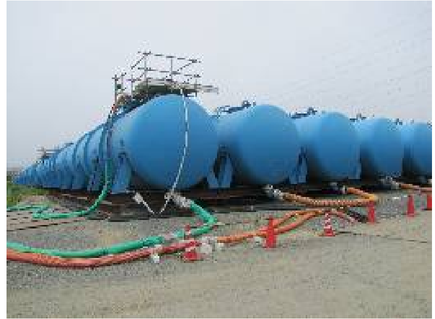
⑭ RO concentrated water storage tank (H1 area) Sep 15, 2011
