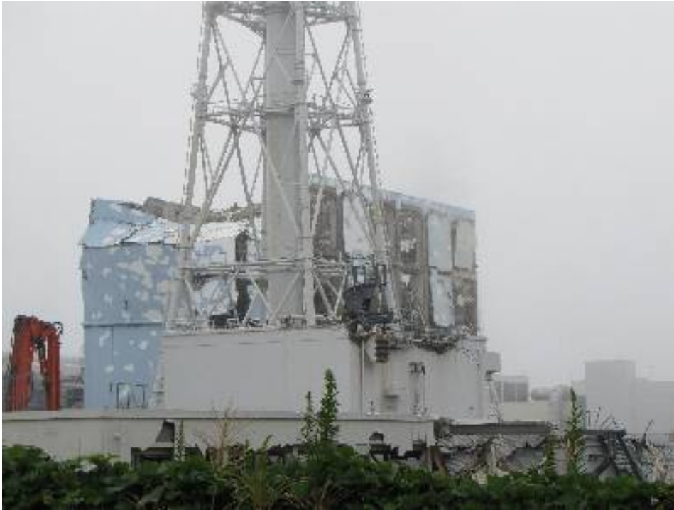
⑨ Overview of a reactor building from western hilltop Sep 15, 2011
