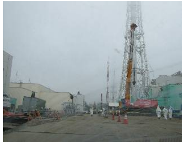
⑩ Rubble collection preparation of a reactor building ~north direction from Unit 4~ Sep 15, 2011
